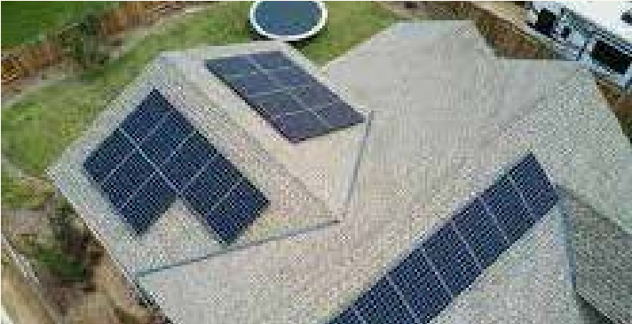
Fig 13 – Solar hot water panels
